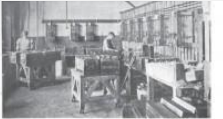
LATERAL BATTERY BANK
