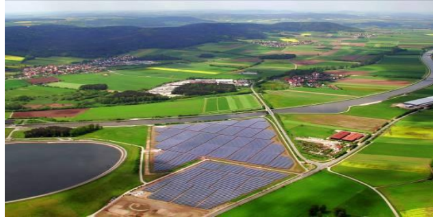
Muehlhausen, Bavaria, Germany, 6 MW SunPower T0 Tracker
